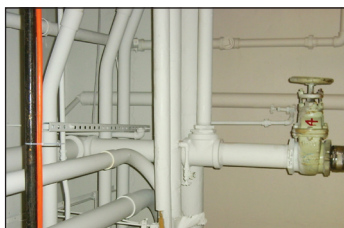
Piping and plumbing systems Photo by John M. Cimbala
